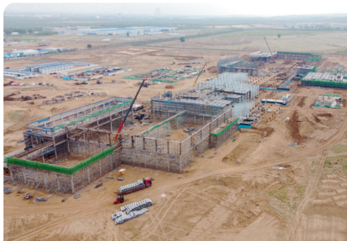
The slaughter and cutting plant for a throughput of 650 pigs per hour was built near the regional capital Hohhot in Inner Mongolia. Photo: Falkenstein
